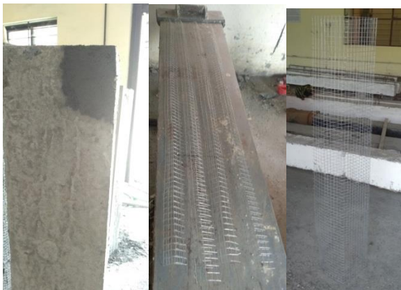
Fig 7: Corners are restored using cement grout and wire mesh cut to required dimension
